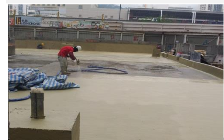
'Fosroc Polyurea WPE' applied on Large Podium Deck with Planters, water features and Vehicles Roads.
